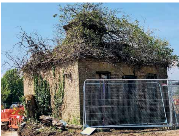
The Proof House at Marsh Gunpowder Works awaiting repairs and restoration summer 2019 ( a grade II listed building).
